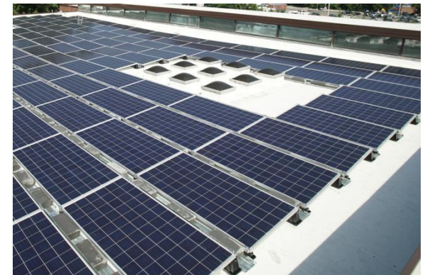
Commercial roof top fixation system
