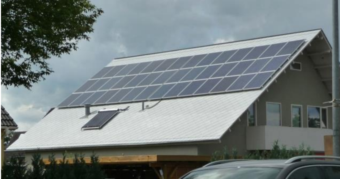
Residential grid-connected PV system (large array) and single solar thermal collector below PV array on a roof in Germany
